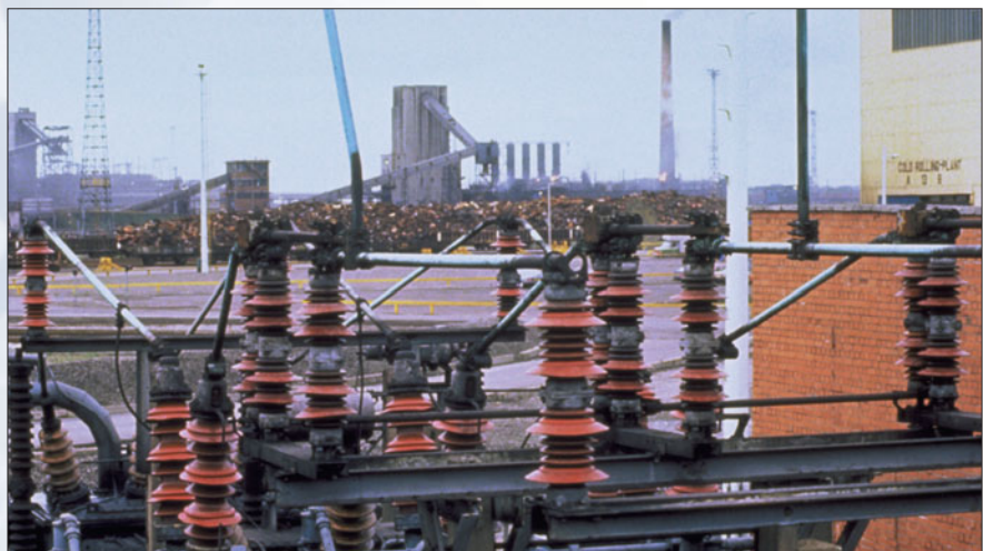
Creepage extenders on 66 kV substation in a heavily polluted marine environment adjacent to a steelworks
