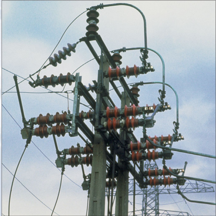
Creepage extenders on 66 kV insulators
